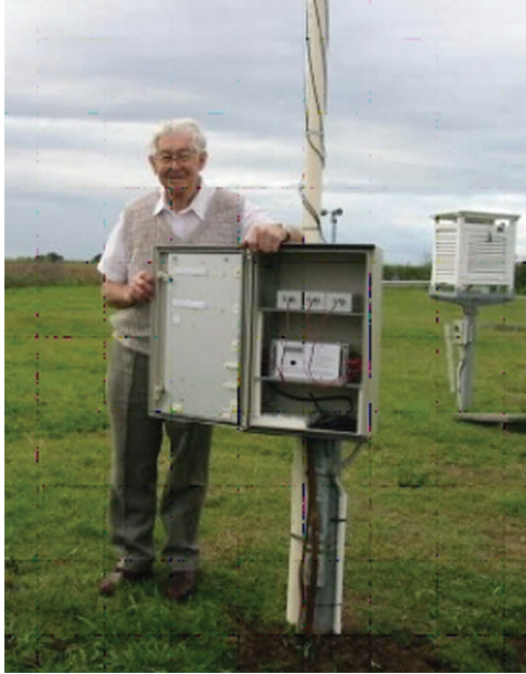
Fig. 8.10 The CGR4 LFCs installed at the Meteorological Station at the Brisbane Airport. The waterproof cabinet contains the CGR4 and three data loggers on a shelf above the CGR4
