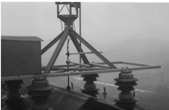
Fig. 9.10 The photo shows the detail of the base of the tower in the Morro do Cachimbo Station
