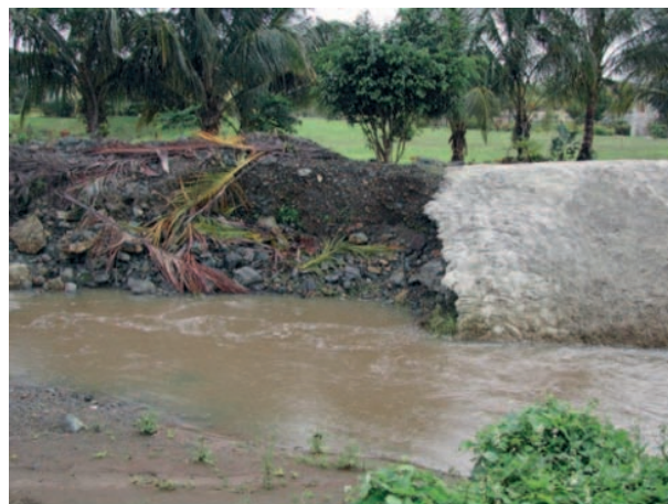
Figure 8 Attempted bank stabilization in Quebrada Maizales, a Puerto Rican stream with suburban and agricultural land use. Note concrete retaining wall, with bank failure on the upstream (left) side of the retaining wall.
