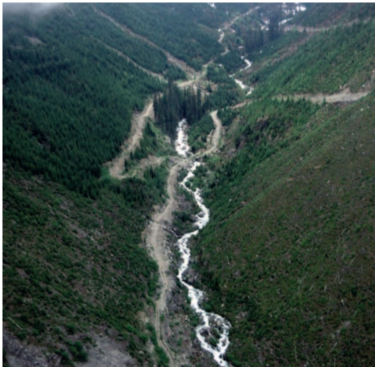
Figure 9 Road construction on moderately steep slopes adjacent to a stream channel, with no buffer strip of undisturbed vegetation in south western British Columbia, Canada, 1999. Photograph by Michael Feller.
