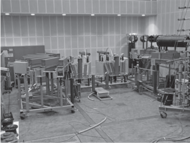
Figure 22.10 Example of an impulse current generator
