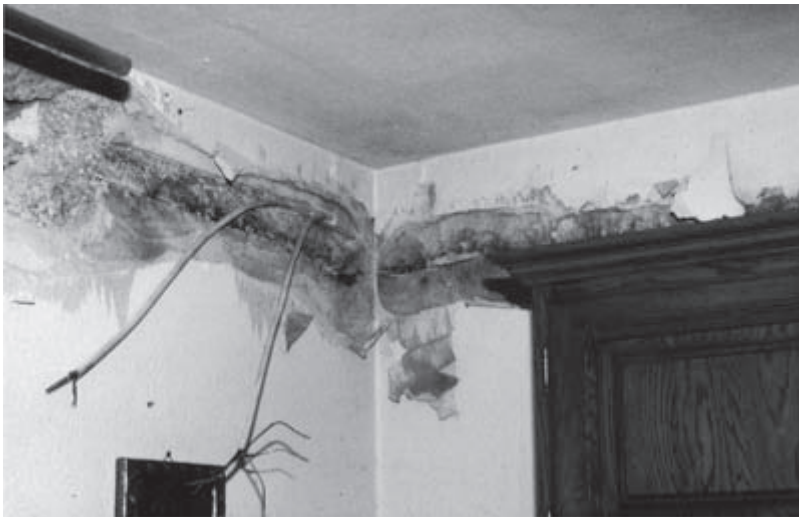
Figure 7.6 Punctures to concealed cables due to lightning strike
