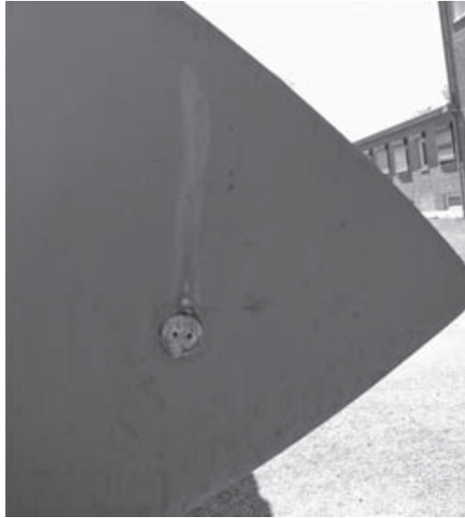
Figure 14.17 Typical scorching of the painted surface of a blade tip on a 40-m blade where lightning has attached to the receptor (photo by the author)
