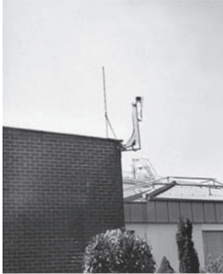
Figure 7.97 Camera for video surveillance in the protective area of the air-termination rod
