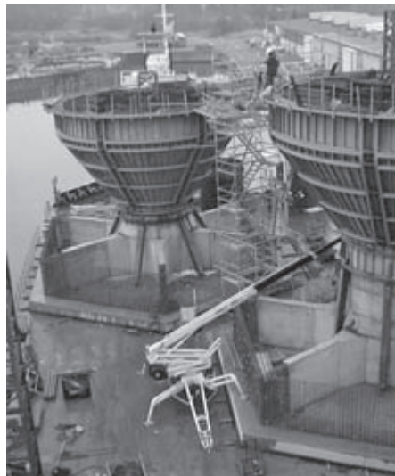
Figure 14.23 Concrete offshore foundations under construction on a barge for later deployment at offshore (photo by the author)
