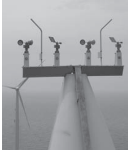
Figure 14.22 Meteorological instruments on an offshore wind turbine protected with lightning air terminals (photo by the author)
