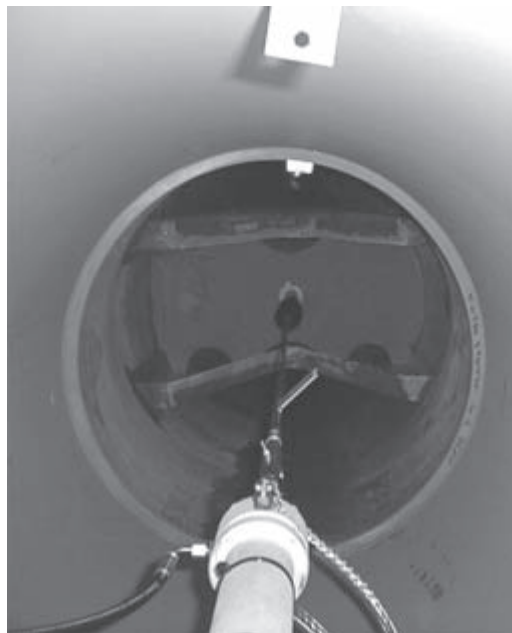
Figure 14.18 A hydraulic piston controlling a steel wire extending into the blade towards the tip air brake. A black hydraulic hose can be seen on the left side of the piston housing and on the right a flexible copper conductor connecting the steel wire and the piston housing (photo by the author).
