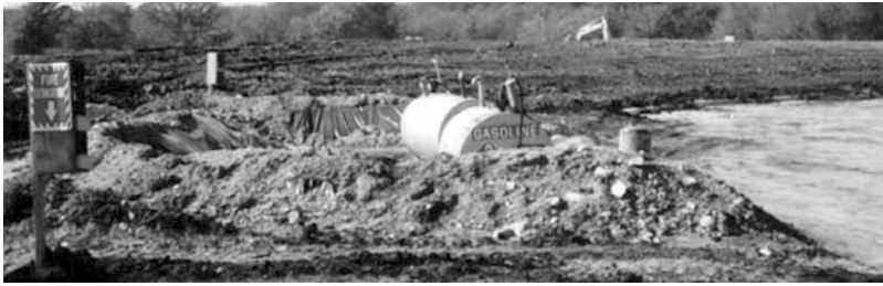
FIGURE 11.1 On-site fuel facility.
